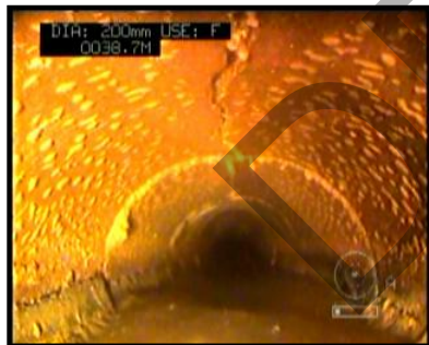
Figure 4.1: Fracture Longitudinal MH 180 to MH 179
