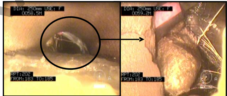
Figure 4.2: Hole in Sewer MH 183 to MH 185
