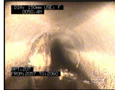
Figure 3.4: Obstruction MH 2057 to MH 2060
