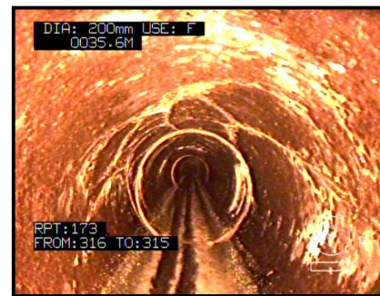
Figure 3.2: Cracks Multiple MH 316 to MH 315
