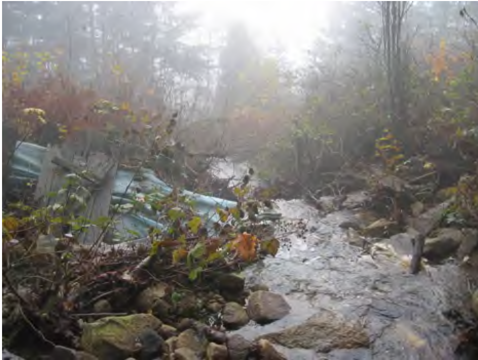
Photo 9: Immediately above Highway 1, the channel of Godman Creek is very steep and would form a fish access barrier; remnants of an old weir structure and fence were found, a short distance downstream of the BC Hydro right-of-way (November 23, 2005).
