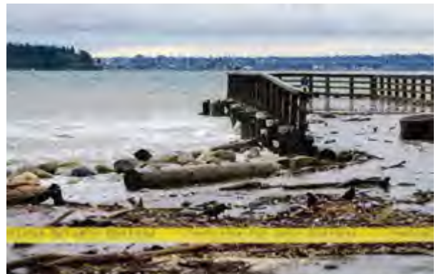
West Vancouver’s waterfront is increasingly prone to flooding during the convergence of high tides and high winds, layered on top of sea level rise. Image: Ambleside, winter 2012
