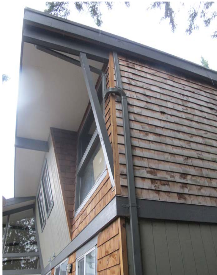
East-facing carport wall now closed with shingle-clad wall to prevent water ingress
