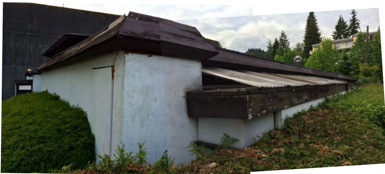
The south east corner of the building showing the warped and split wood wall caps, fibreglass panels cover the courtyard. Plant growth is right up against the building walls
