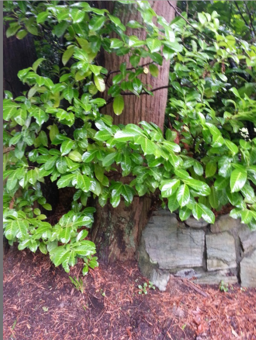
Photo 2: The existing rock wall is embedded into the trees trunk.
