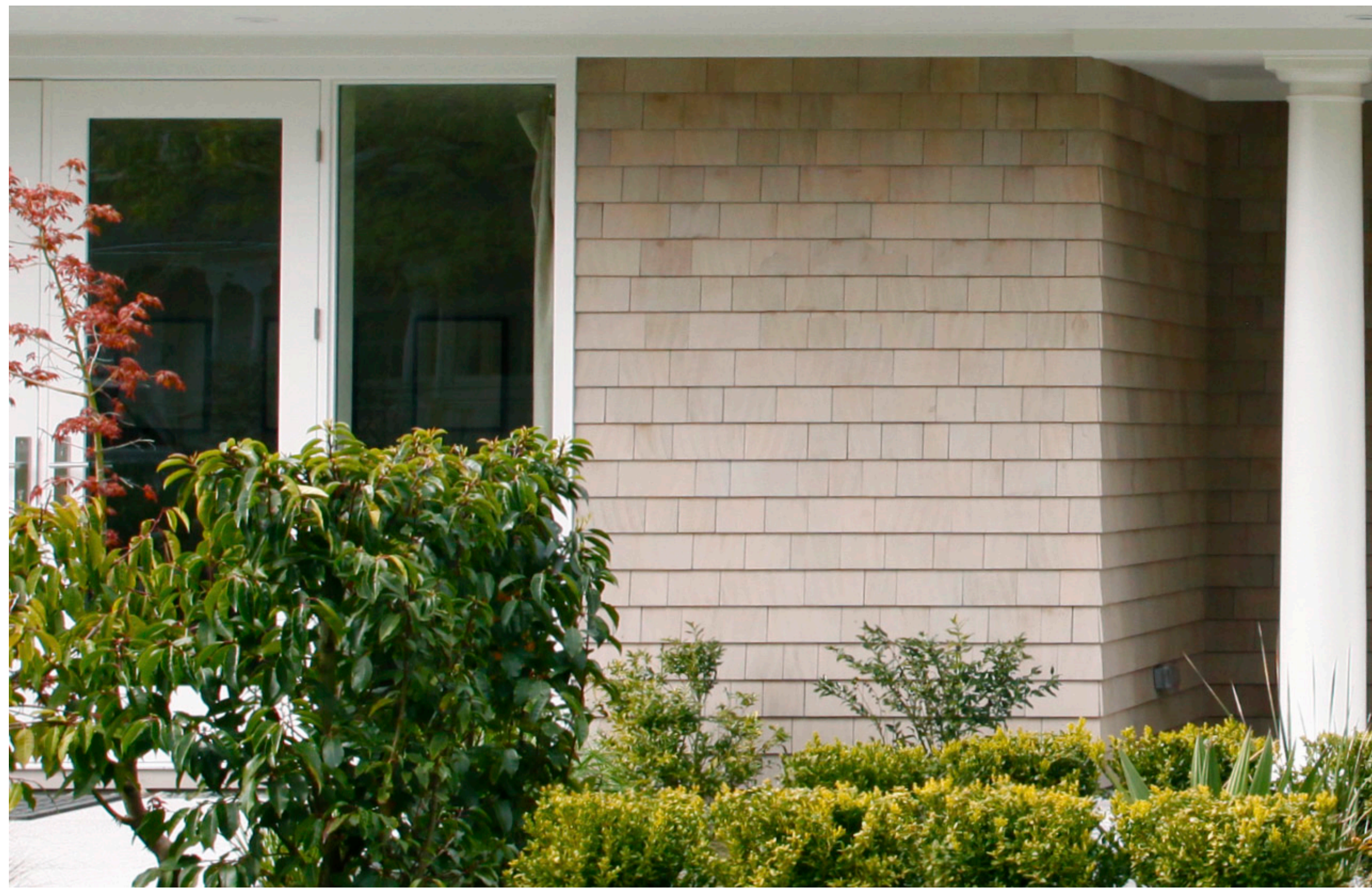
13 Wall shingles will be # 1 boxed "perfection" resawn and rebuted Western red cedar shingles stained with General Paint "Glutted" colour semi-solid stain, 5" to weather. The roof will be quaternian treated resawn western red cedar, 5 1/2" to weather
