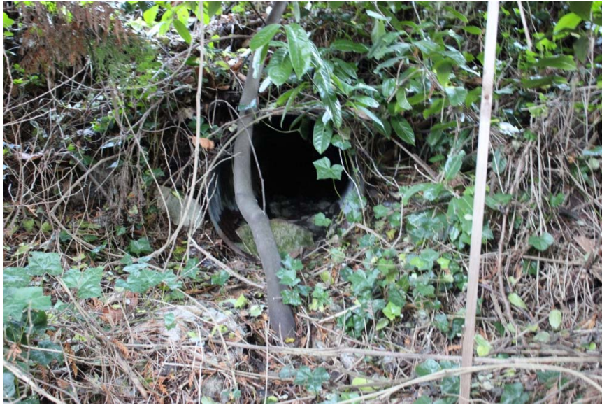
Photo 1. Unnamed watercourse originates at culvert outlet on property at Marine Drive. View looking upstream (North) towards Marine Drive.
