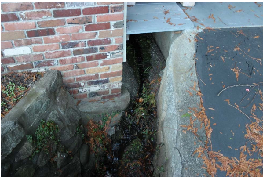
Photo 6. Outlet of concrete lined channel under existing deck. View looking upstream towards existing structure.
