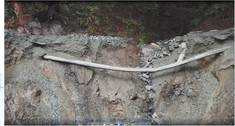
Subsequent Landslide – January 13
