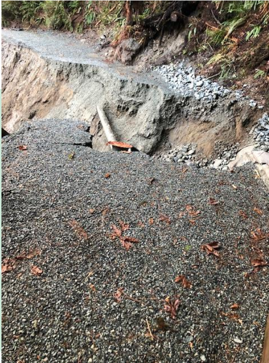
Initial Landslide – January 6
